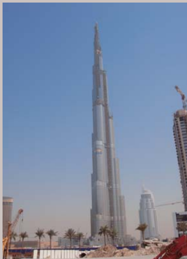
The 800m Burj Dubai Tower under construction in the emirate of Dubai in the UAE.
